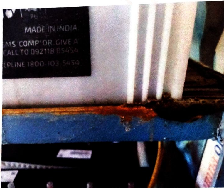
Figure 13 - Galvanic reaction causing damage to battery life.
